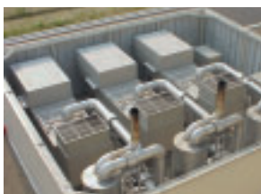
Cogeneration systems (Koriyama Plant)
