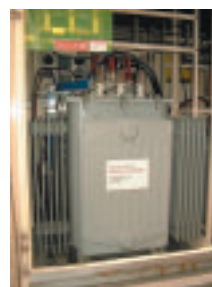
Electrical substation facility at the Sagami Operation Center, where PCB contamination was found
