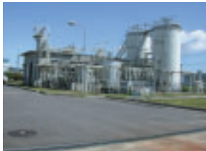
Wastewater treatment facilities (Koriyama Plant)
