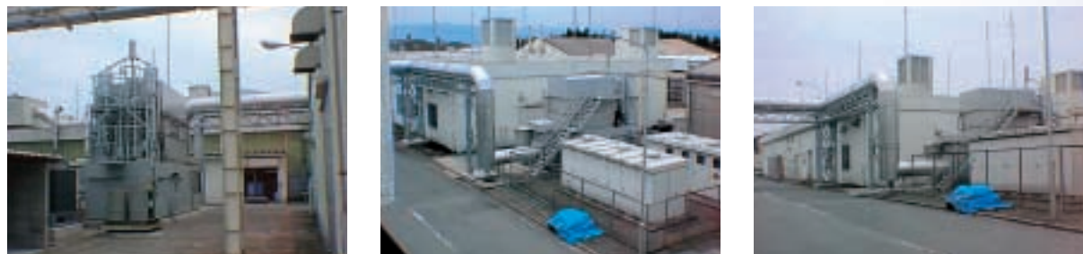
External view of the deodorization equipment installed at the Aso Plant
