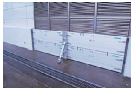
Installed water bars at the entrances to buildings to reduce flooding risks (Sagami Operation Center)
