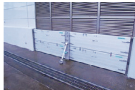
Installed water bars at the entrances to buildings to reduce flooding risks (Sagami Operation Center)
