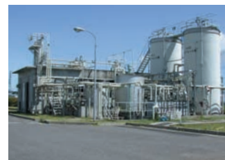
Methane fermentation wastewater treatment facilities
