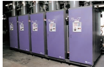
Natural gas boilers
